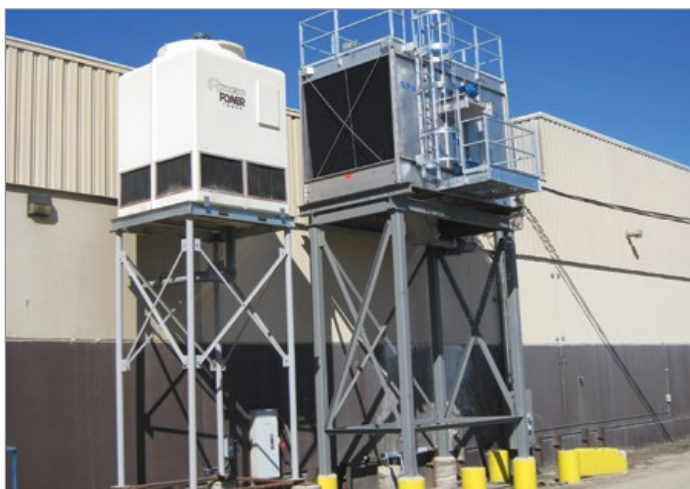
New cooling tower and tower auxiliary equipment.
